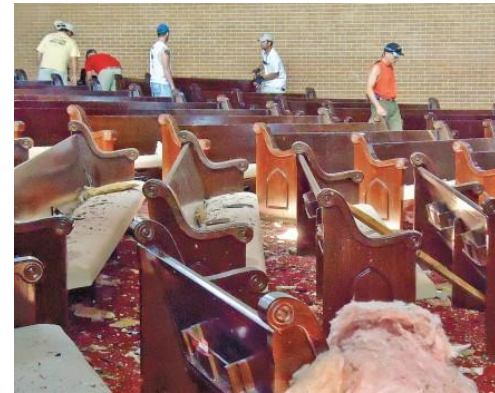
PHOTO BY JEREMY D. SMITH - CENTRAL CHURCH OF CHRIST - Members survey tornado damage inside the Central Church of Christ auditorium. Some gather songbooks and begin removing pews.
